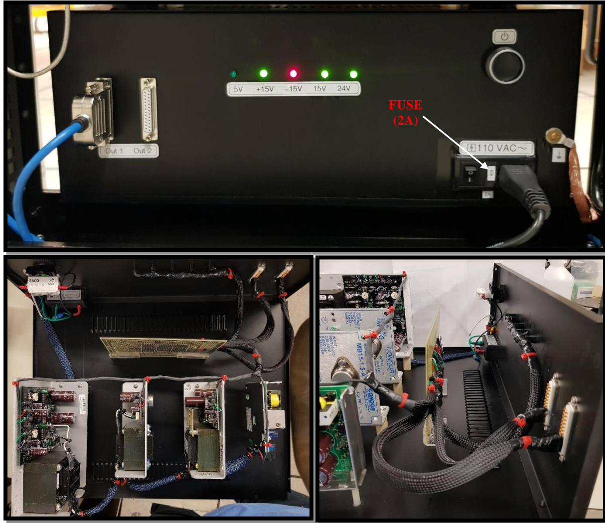
Figure 2.1: Q-meter and Yale-Card power supply box
