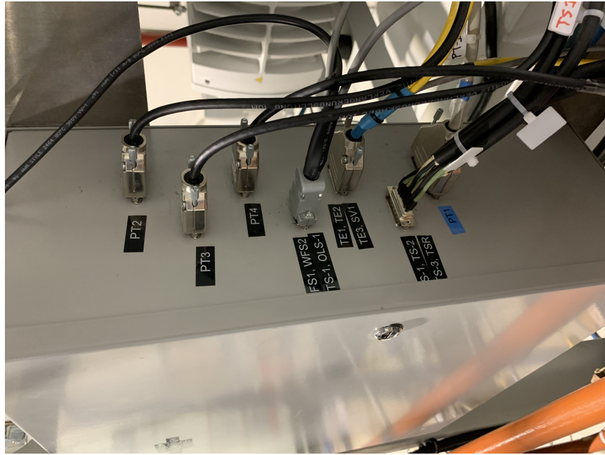
Figure 9: 24 VDC feedthrough panel
