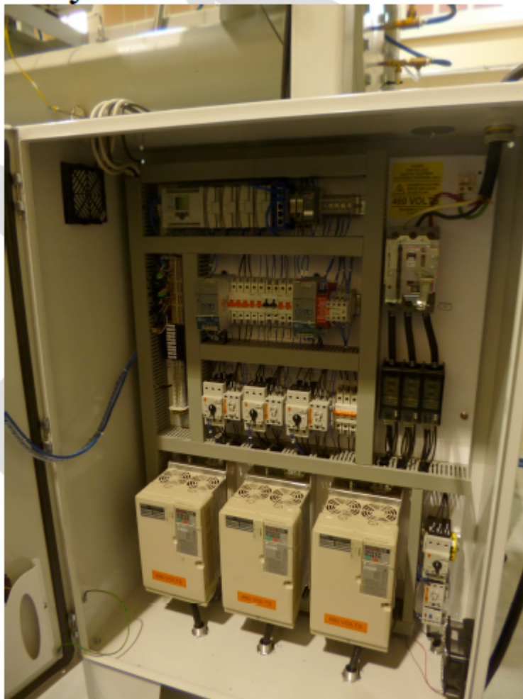
Figure 14: Electrical control panel
