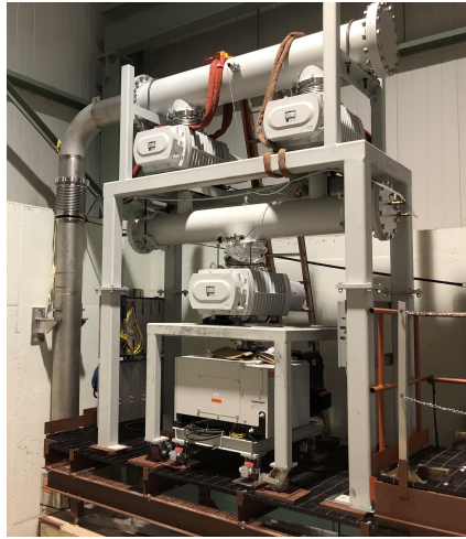
Figure 1: Image of Root Pump Stack installed at NM4
